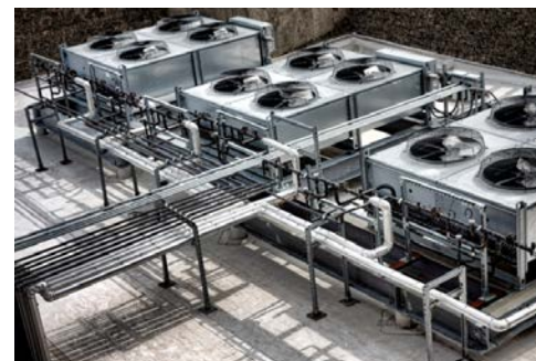
Buildings and infrastructure, such as HVAC units, can serve as energy storage systems.
