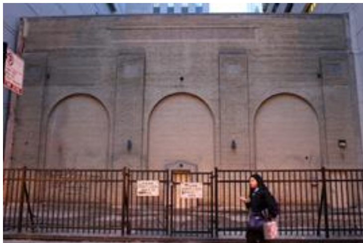
Figure 8.13. An enclosed substation (note indoor design blends in with its surroundings).
