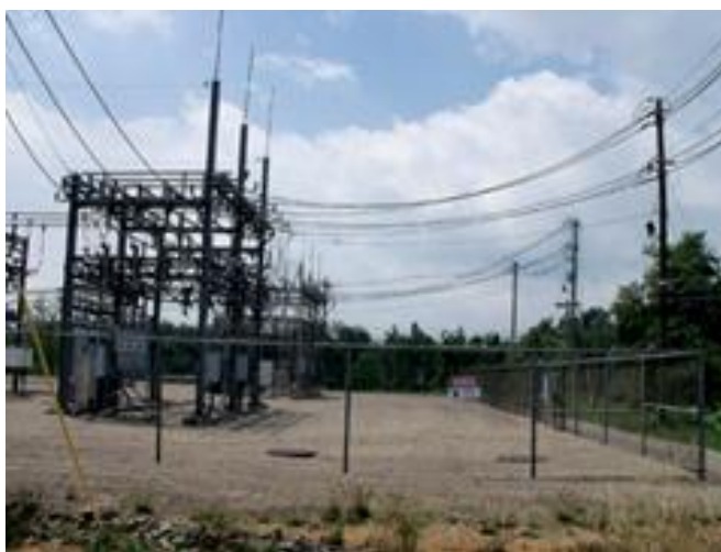
Figure 8.14. An open-air substation (note absence of secondary containment).
